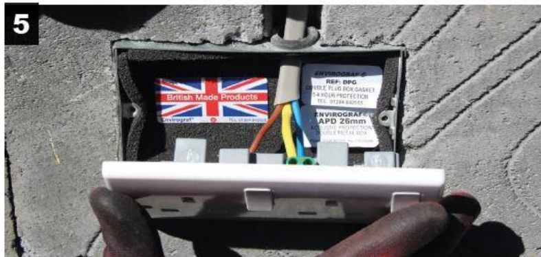
5 Job done. You now have fully fire and acoustic protected metal box.
