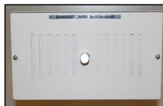
Vent in closed position
